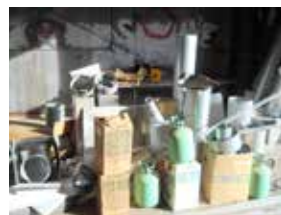
Heating Air Conditioning Duct Work and other Items
